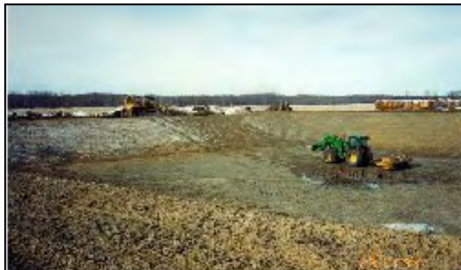
A properly designed, constructed and operated manure storage facility is insurance against spillage.
